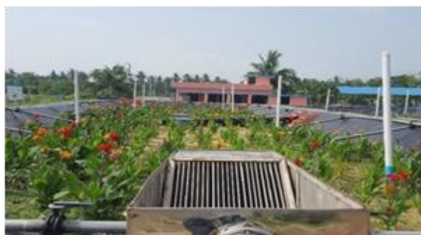
Constructed wetland (pre-treatment)
