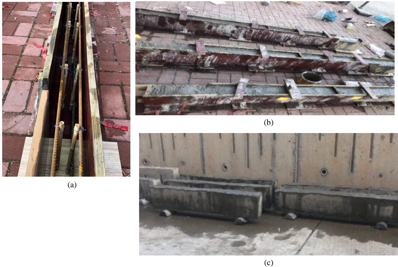
Figure 5. Different stages of the work: (a) caging, (b) casting concrete, and (c) curing the beams
