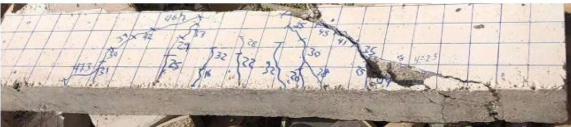
d) The crack pattern of the beam 3Q12
